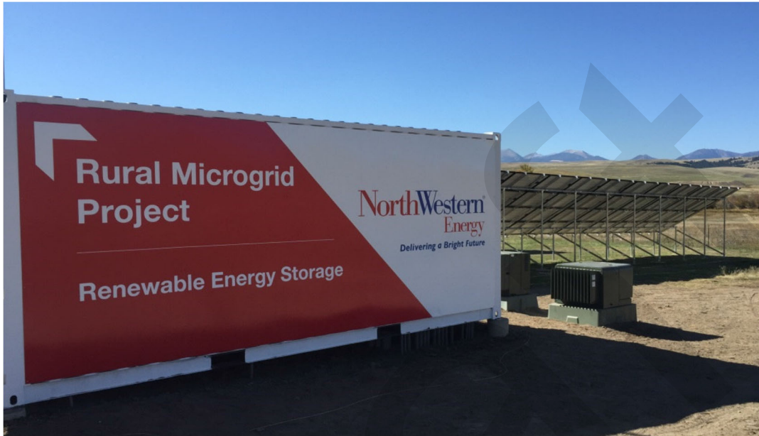
Figure 8-2. Deer Lodge Microgrid Solar PV Array and Containers
