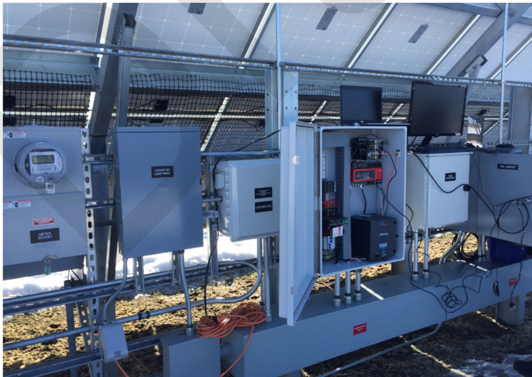
Figure 8-5. Bozeman Solar Microgrid Container Boxes and Controllers
