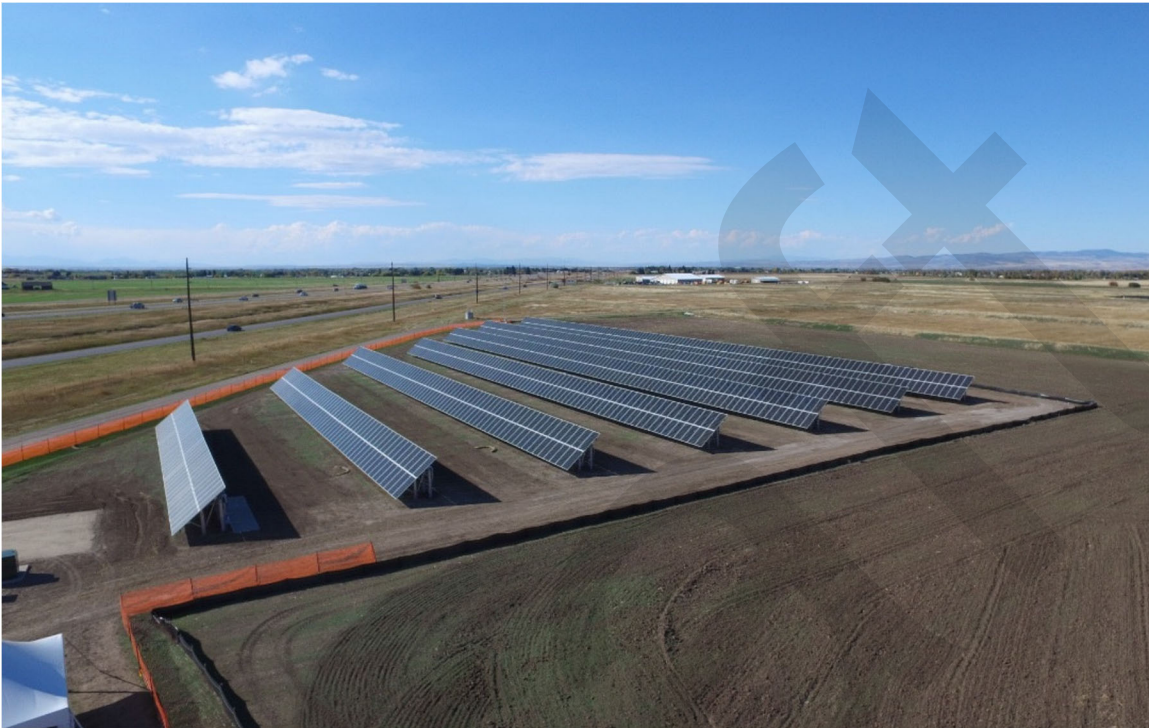
Figure 8-6. Bozeman Solar Microgrid 380 kilowatt Array
