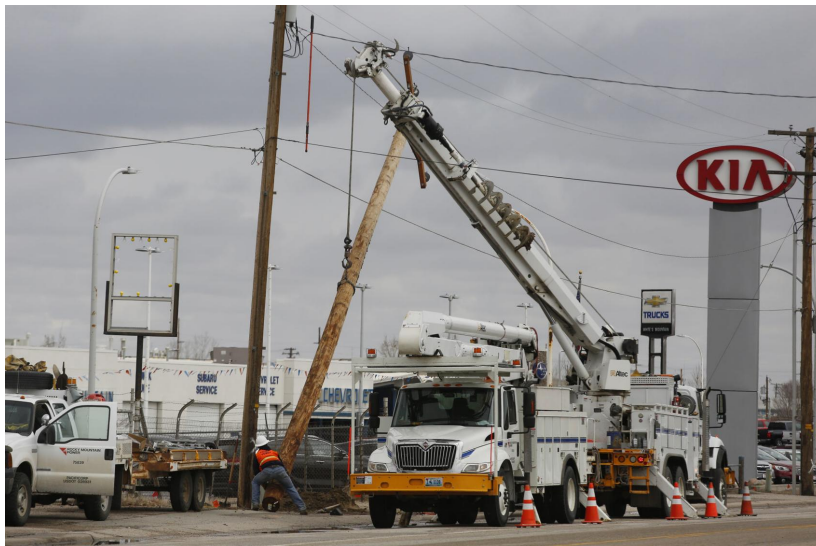
Linemen from Rocky Mountain Power install a new utility pole in April 2017 on East Yellowstone Highway in Casper. A new bill could force utilities to sell their coal plants instead of closing them.
