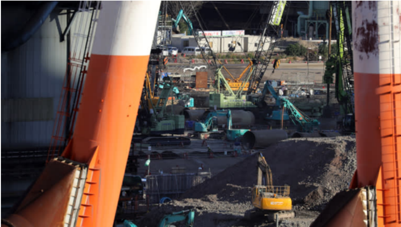
Kobe Steel is expanding its coal-fired power plant in Kobe, which is expected to double the plant's emissions. (Photo by Ken Kobayashi)
