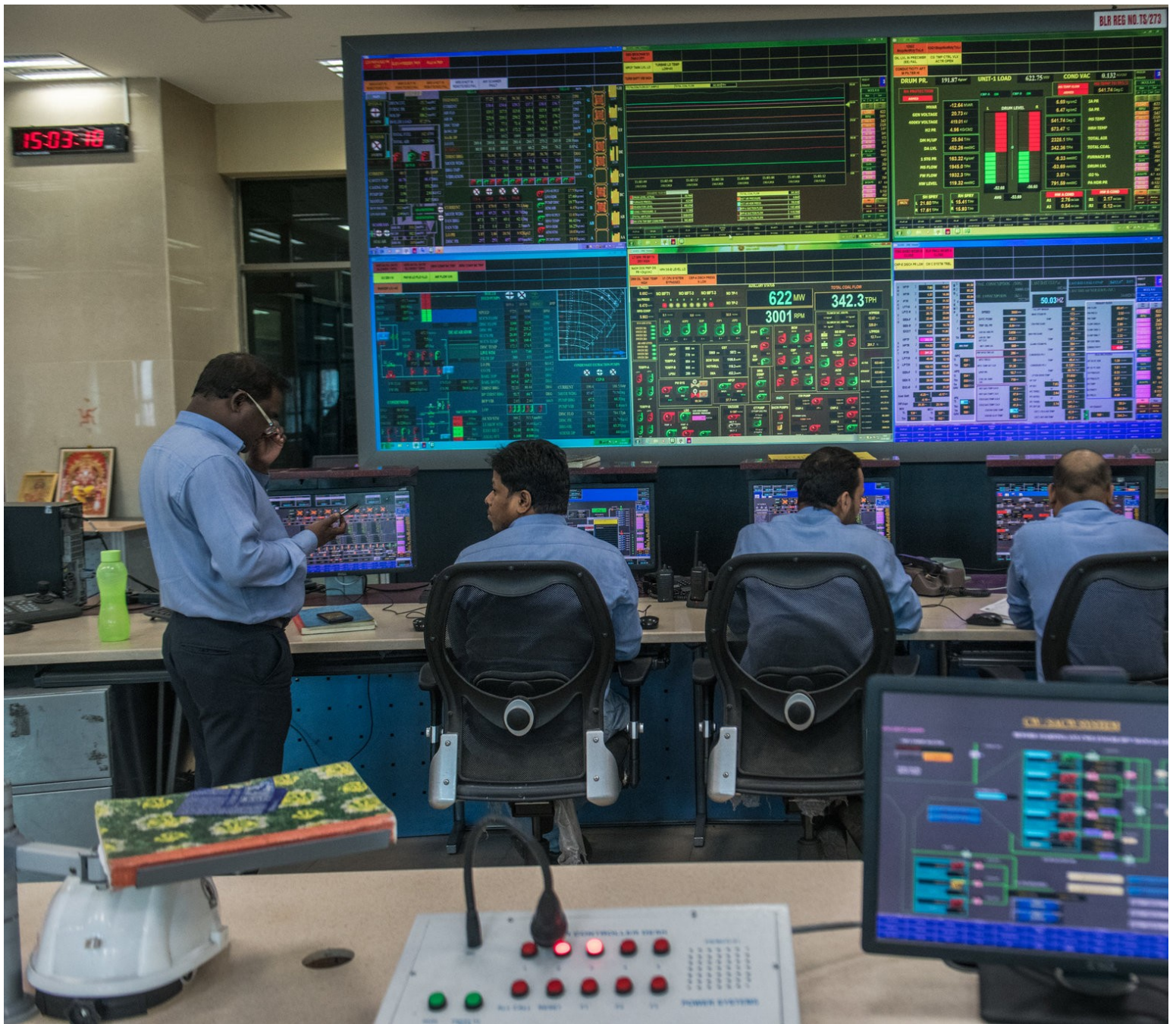
The control room of a power plant in Mancherial, Telangana. Rebecca Conway for The New York Times
