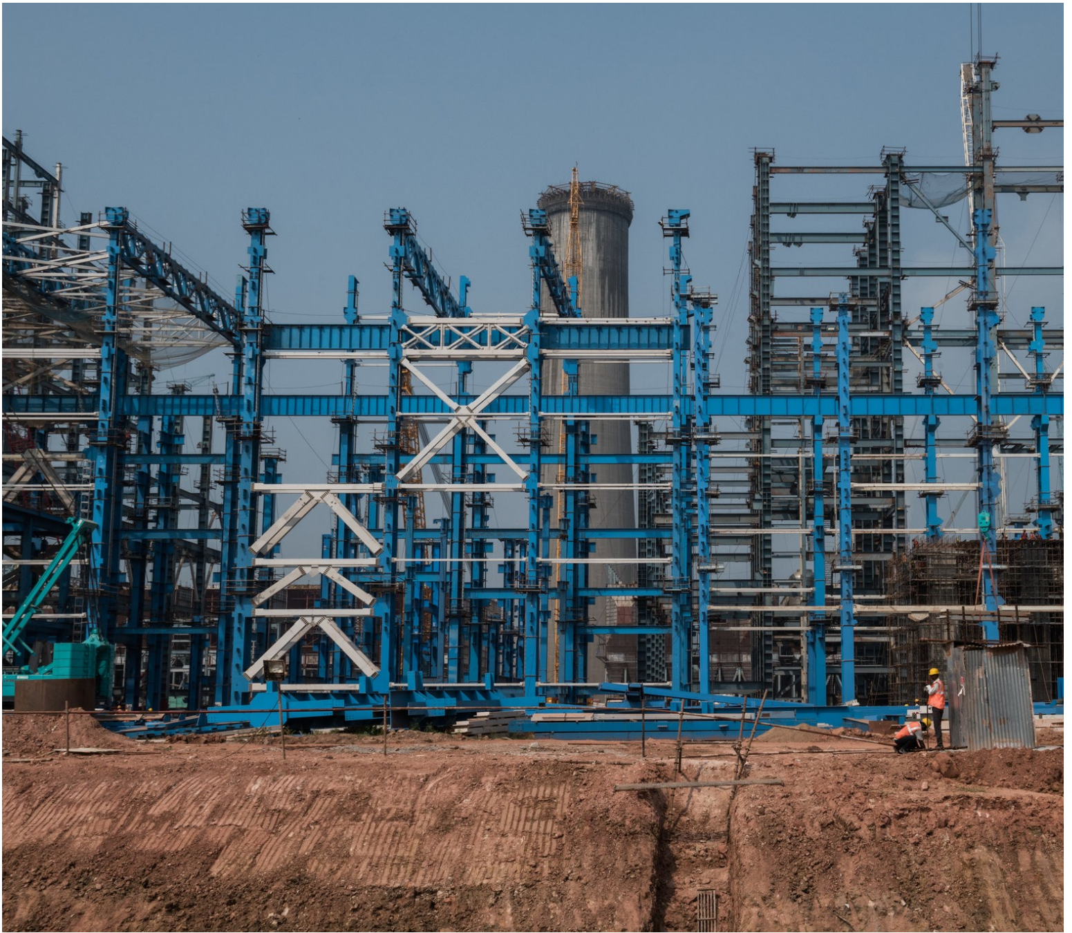
A coal-fired power plant under construction in Ramagundam, Telangana State, India. Rebecca Conway for The New York Times
