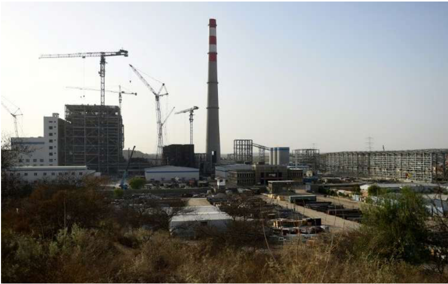
Towering chimneys emerge from the sand dunes of the Thar desert as Pakistani and Chinese workers toil away on a 660-megawatt power plant
